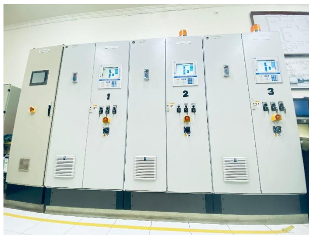
Fig. 9. CCR control panel PLTMG Bawean
