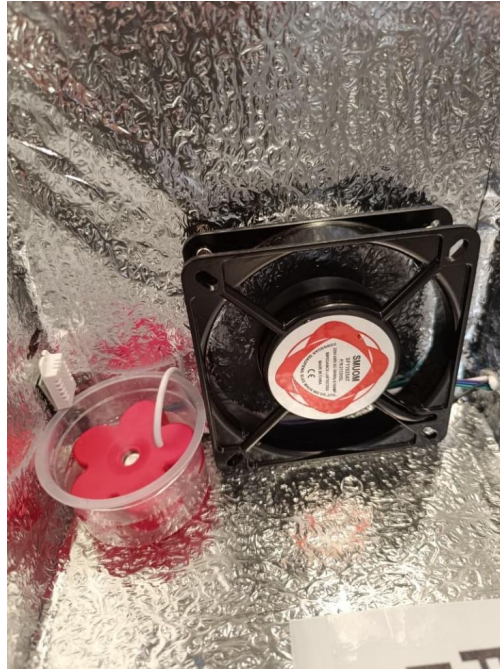
Fig. 5. Ventilation fan, humidifier, and DHT22 sensor in operation
